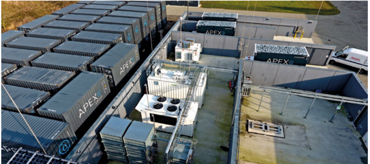
The buffer storage tanks hold the hydrogen ready for refueling at 350 bar (truck) or 700 bar (car)
